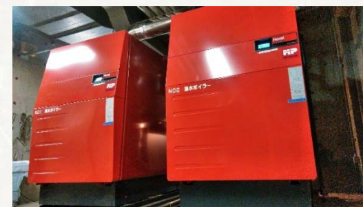
Implementation of large-scale renewal by utilizing subsidies: Energy costs were reduced as a result of making the boiler operate on gas instead of heavy oil
